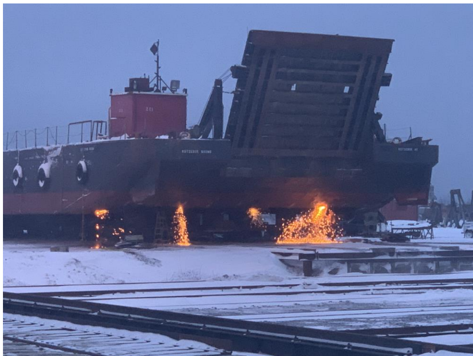
The Barge Kotzebue Sound Gets Repair Work Done at Seward Shipyard (Photo Courtesy JAG Alaska, Inc.)
